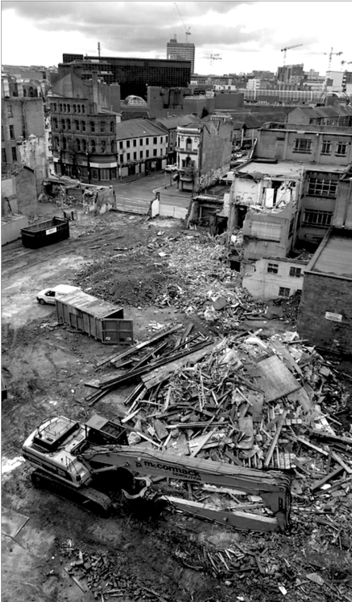
Figure 4-25 Demolition of historic city centre buildings to make way for student services (leslie, 2017)
